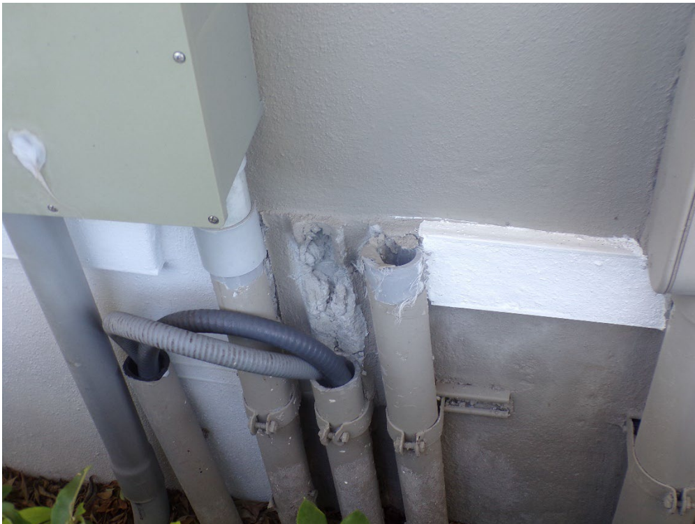
Unsealed electrical and poorly finished stucco.
