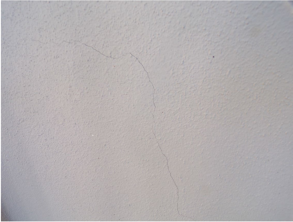
View of typical stucco crack on side of clubhouse.
