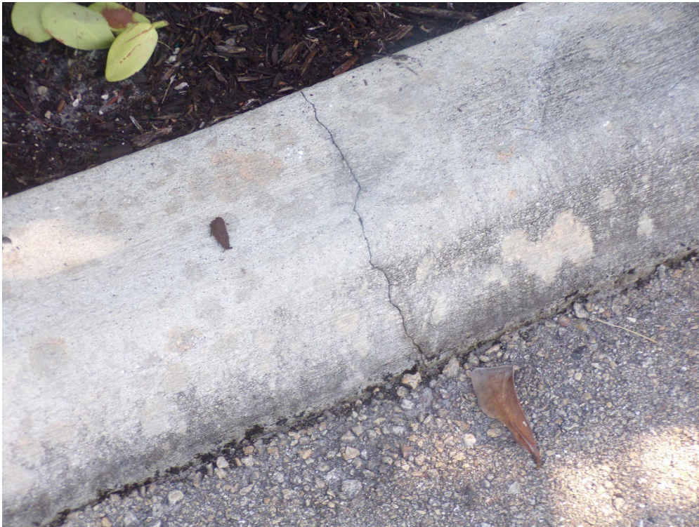
View of typical concrete curb crack.
