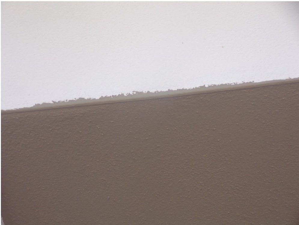
View of sloppy paint job on clubhouse edge.
