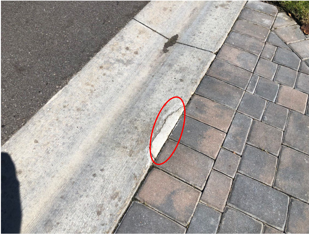
View of crack on concrete valley gutter.
