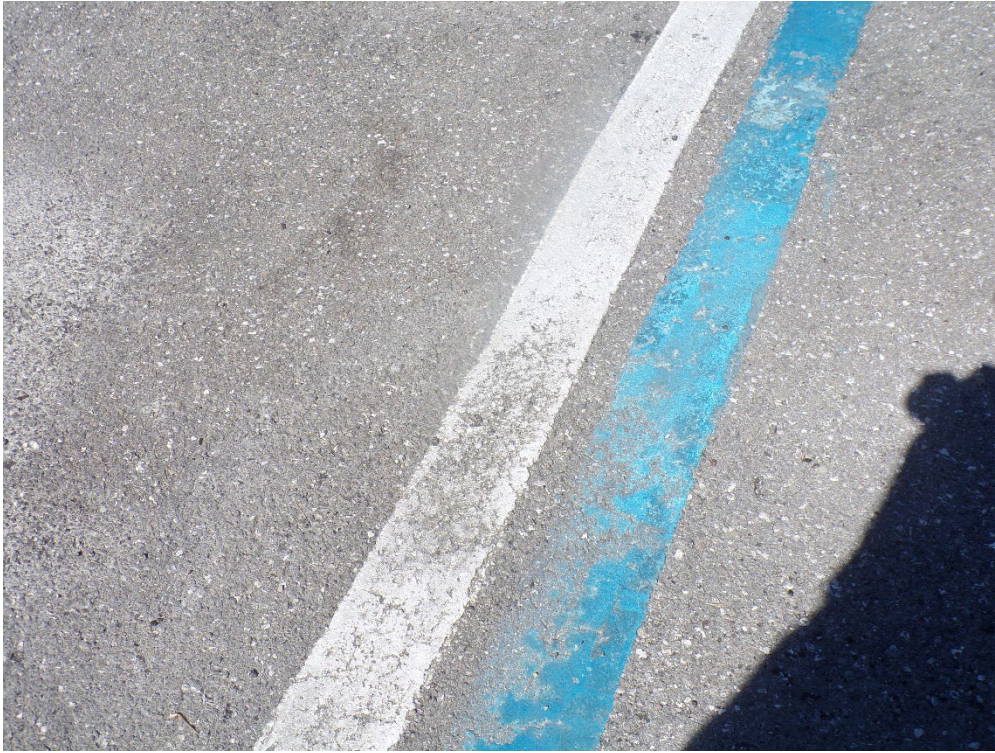
View of fading paint stripes on parking spaces.
