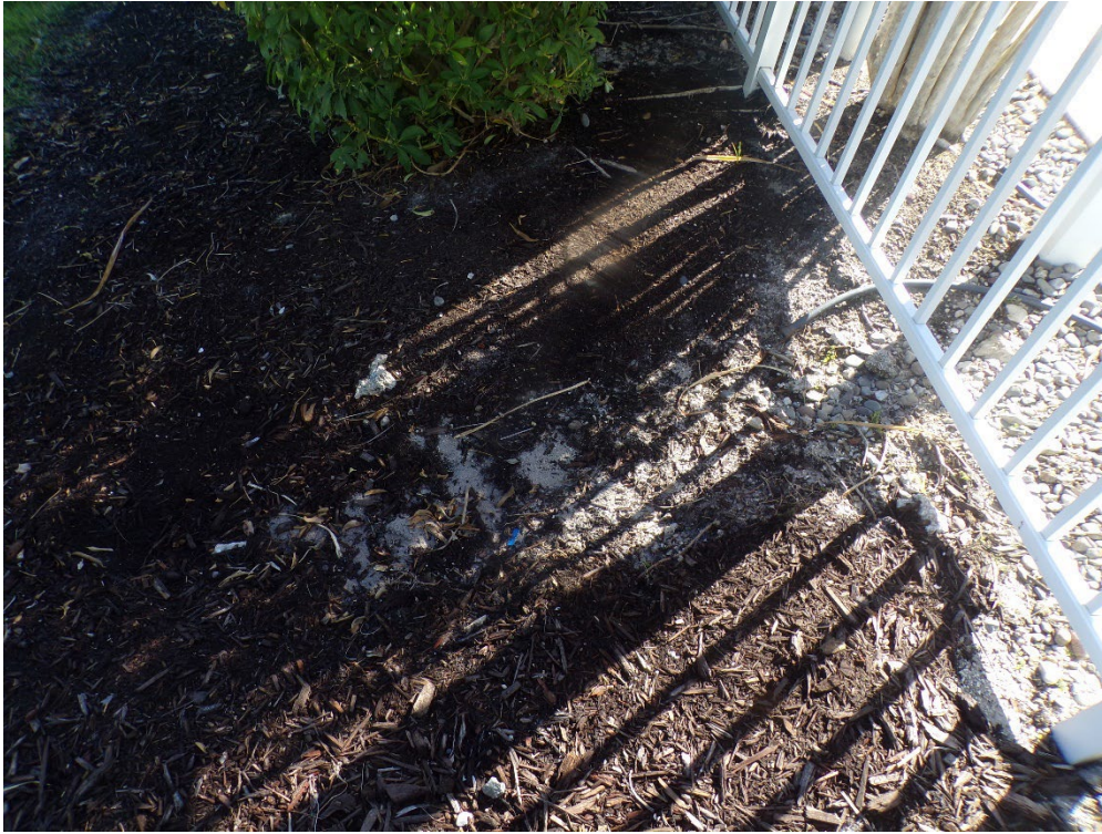
View of minor soil washout next to pool area.
