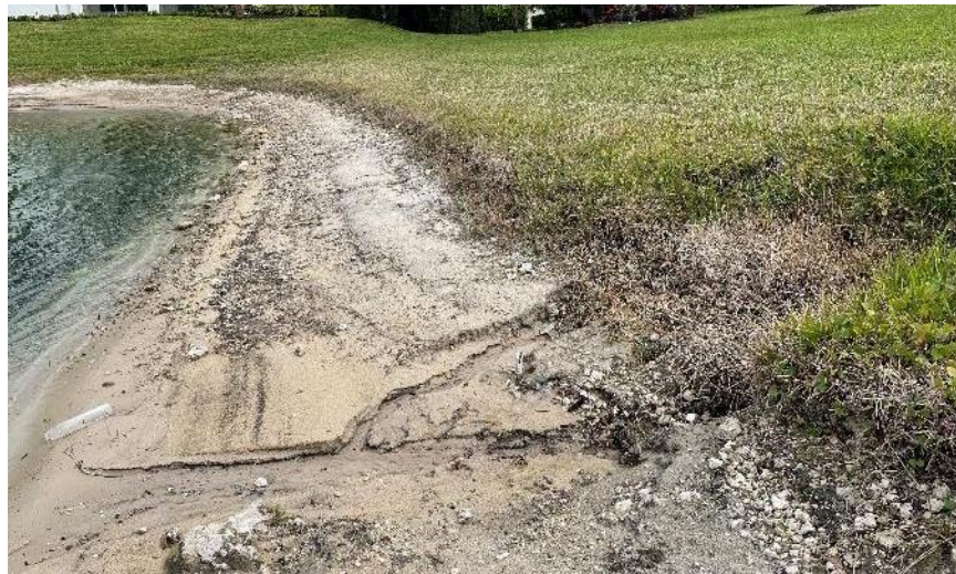
Photo 2.7-5: Isolated erosion at south side of Lake 2B
