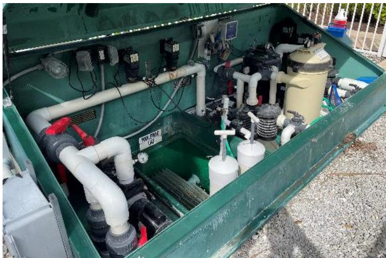
Photo 2.4.4-1: Pool and spa equipment
