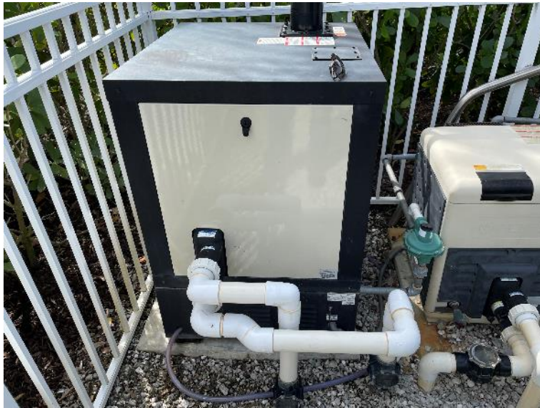
Photo 2.4.4-2: Pool and spa heater
