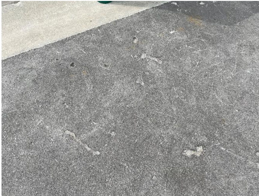
Photo 2.5.1-2: Surface damage at Sawyers Hill Road
