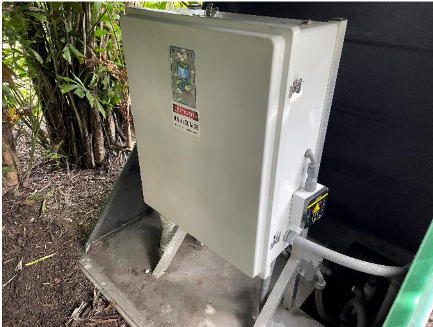
Photo 2.8-2: Irrigation pumping station equipment
