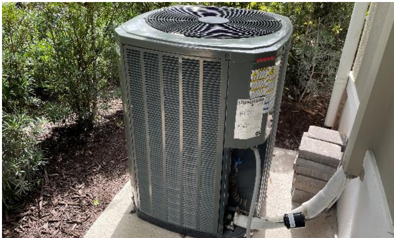
Photo 2.3.5-1: Air conditioning condensor at clubhouse
