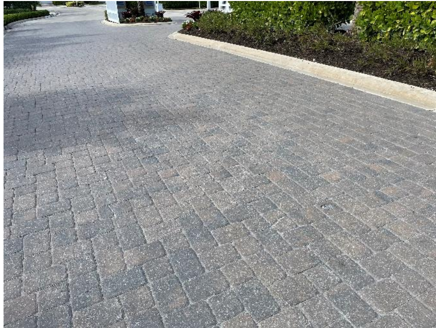
Photo 2.5.2-1: General condition of pavers at entrance
