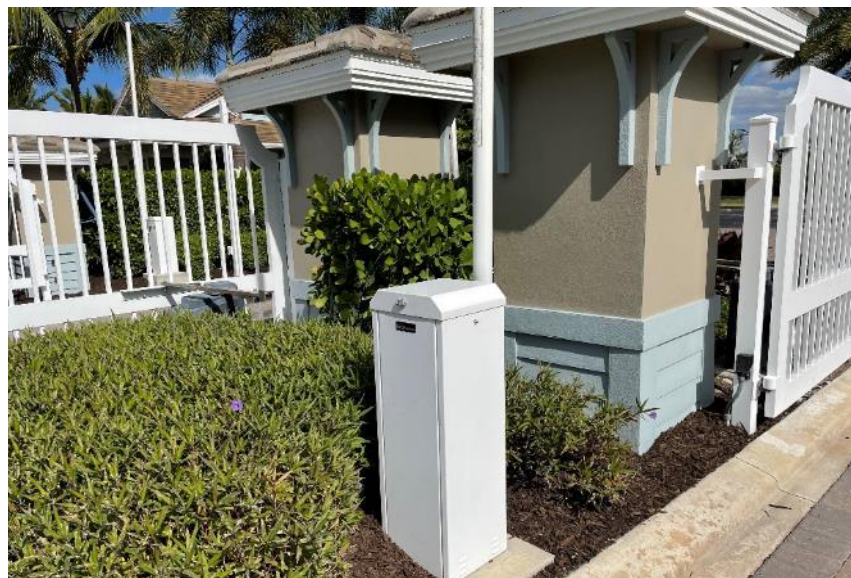
Photo 2.2-3: General view of barrier arm
