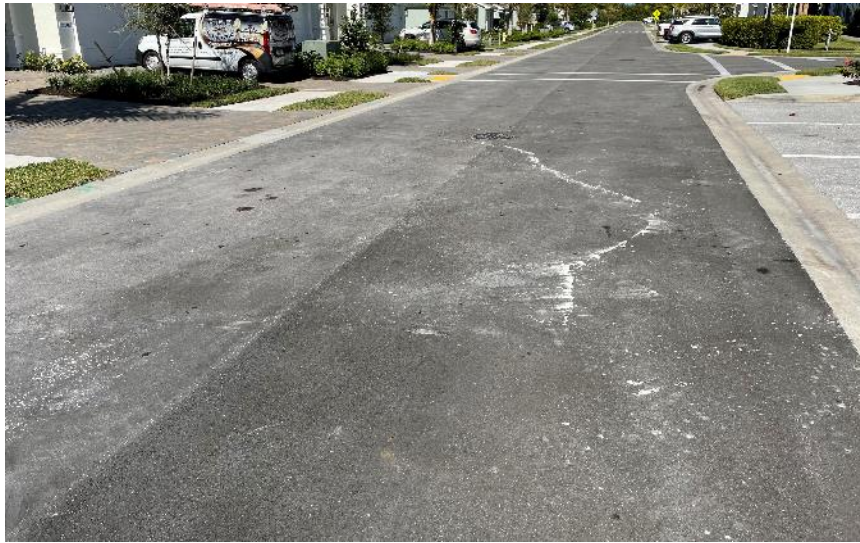
Photo 2.5.1-3: Surface staining at Sawyers Hill Road
