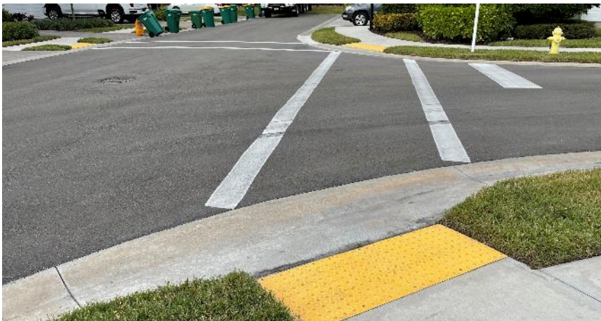
Photo 2.5.1-5: General view asphalt pavement at intersection of Sheen Lane and Sawyers Hill Road
