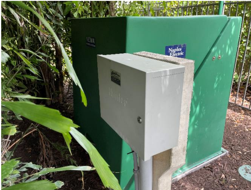
Photo 2.8-1: Irrigation pumping station and controller
