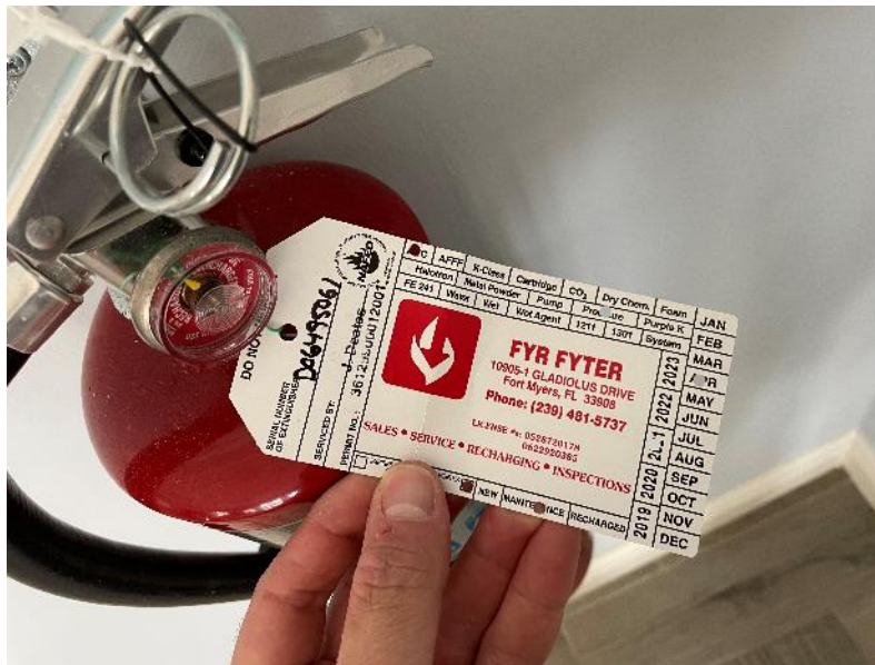
Photo 2.3.6-1: Current inspection tag on fire extinguisher
